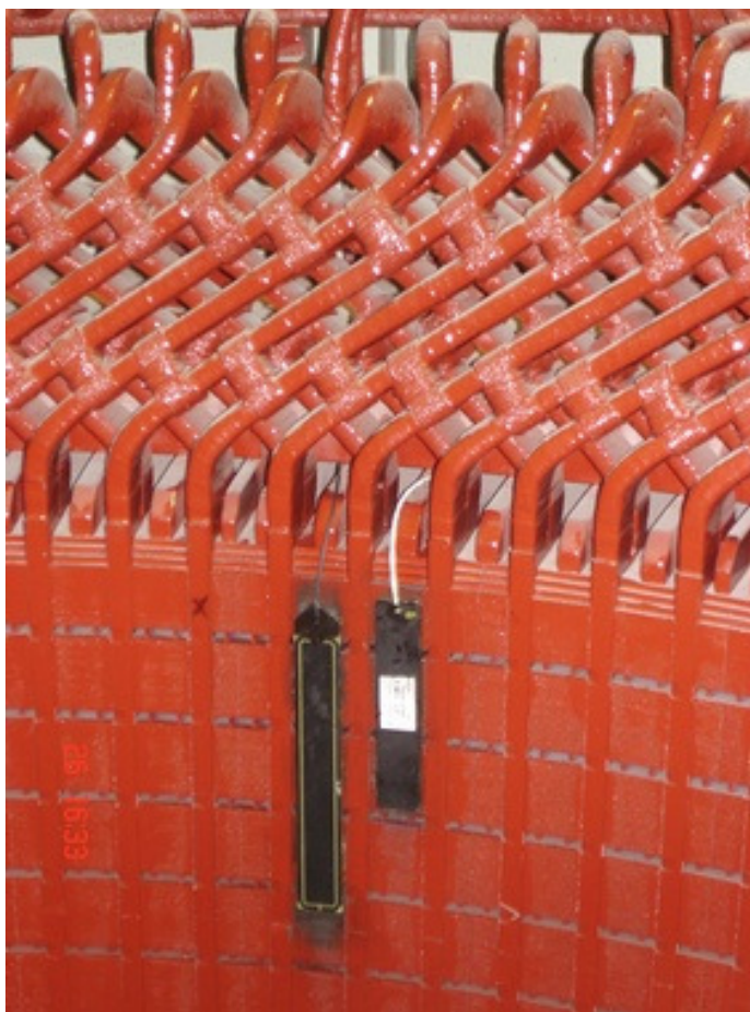
Figure 12. AGSP sensor probe installed at stator surface (AGS sensor pictured on the left, magnetic field sensor on the right side)
